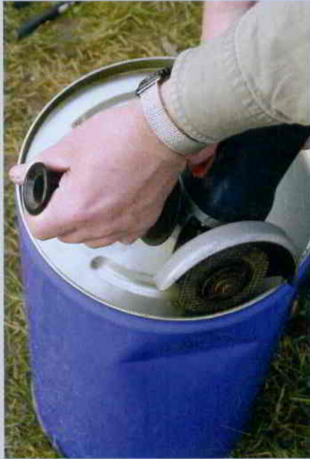
STEP 1. Cut the top out of a drum with an angle grinder, leaving the top rim intact for strength. Clean out the drum if needed. Make a clip-on top from a sheet of metal approx 5cm wider than the drum, by folding over approx 2.5cm each side.
