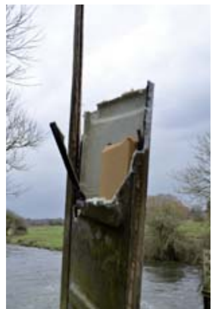
The floods have damaged some of our equipment and large-scale repairs are now in progress.
