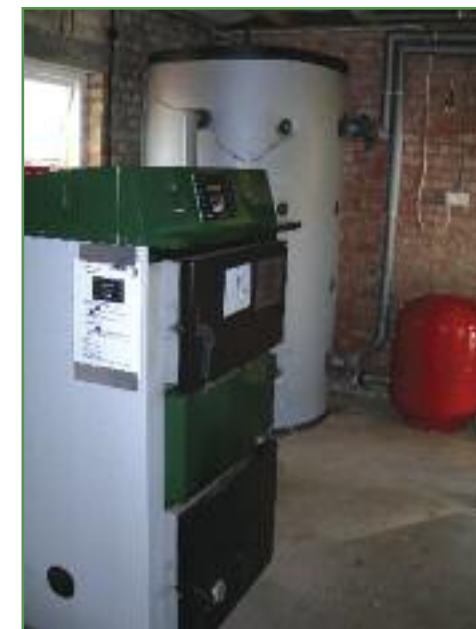
A modern high-tech woodfuel heating system for a local four bedroom house.
