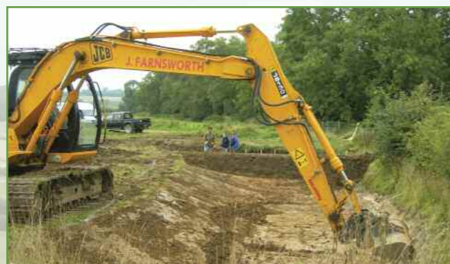
Tilton contractor John Farnsworth excavates a prototype field corner wetland for new water quality research at Loddington.
